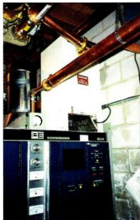
Reject load above KBSU's Broadcast Electronics FM-10A transmitter.
